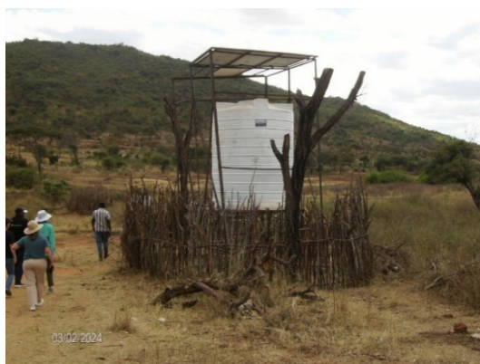
An electric vertical turbine pumps water to this storage tank; note four solar panels at the top.
