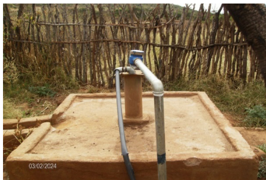
This well is equipped with a solar-powered submersible pump and its discharge is piped to a small, elevated tank.
