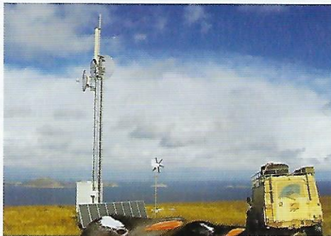
The network's remote telecom sites will be powered primarily by renewable energy such as wind turbines and solar panels.
