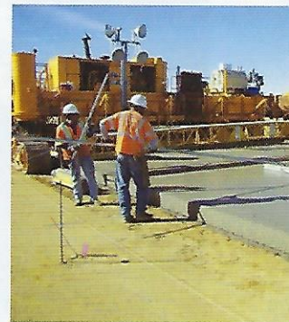
Workers smooth out newly laid concrete on the temporary runway at Edwards Air Force Base in California. The runway's surface can only vary by one-eighth of an inch (0.32 centimeter) over the 7 total miles (11.3 kilometers) of runway, taxiway, and access area.
