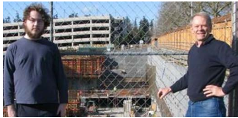
John Dennison and Art Storbo discuss excavation and concrete construction for Bellevue Hospital garage
