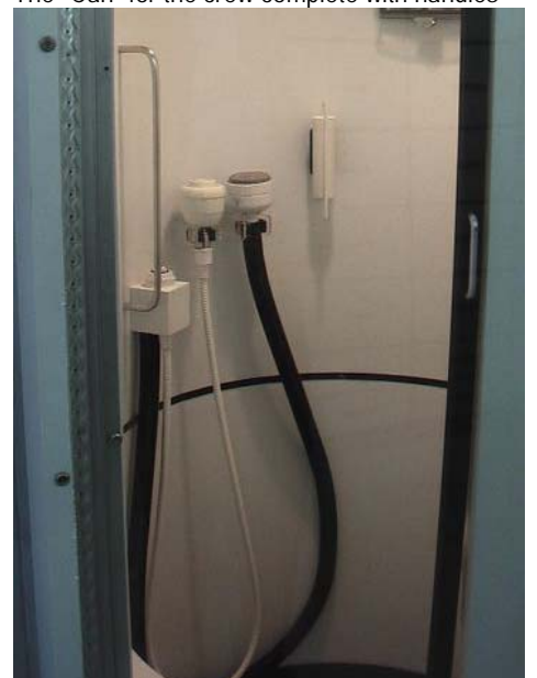
Shower for the crew
