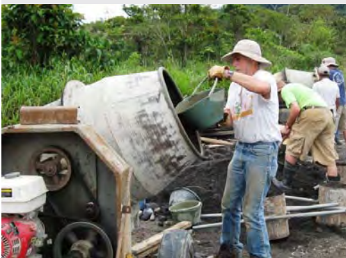
Dennis mixing concrete in Ecuador, where he joined others preparing the site for La Casa de Fe
