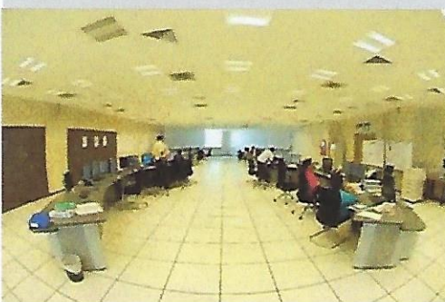
The Changi water reclamation plant control room
